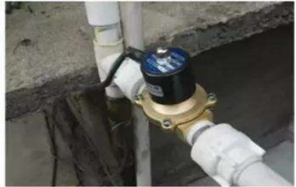
pipeline water control
